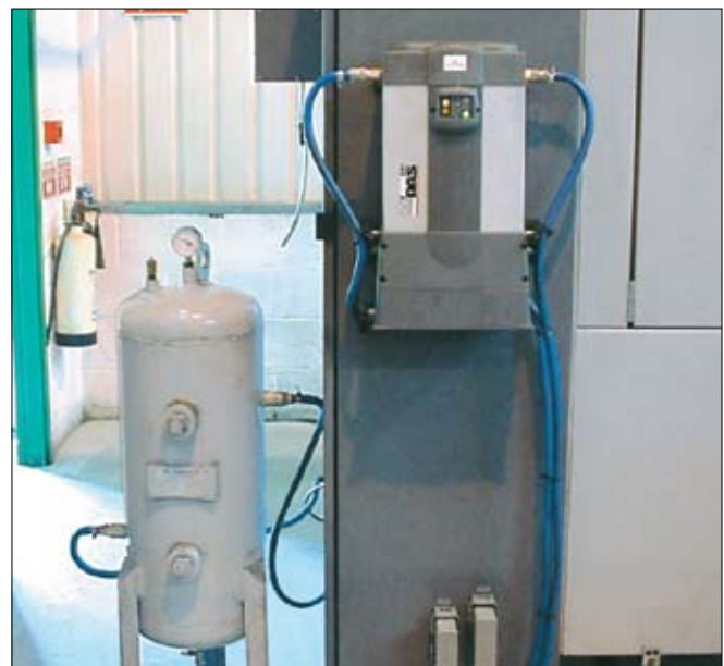
A Regenerative Desiccant Dryer System Installed to Supply Control Air for a CNC Machining Center.
